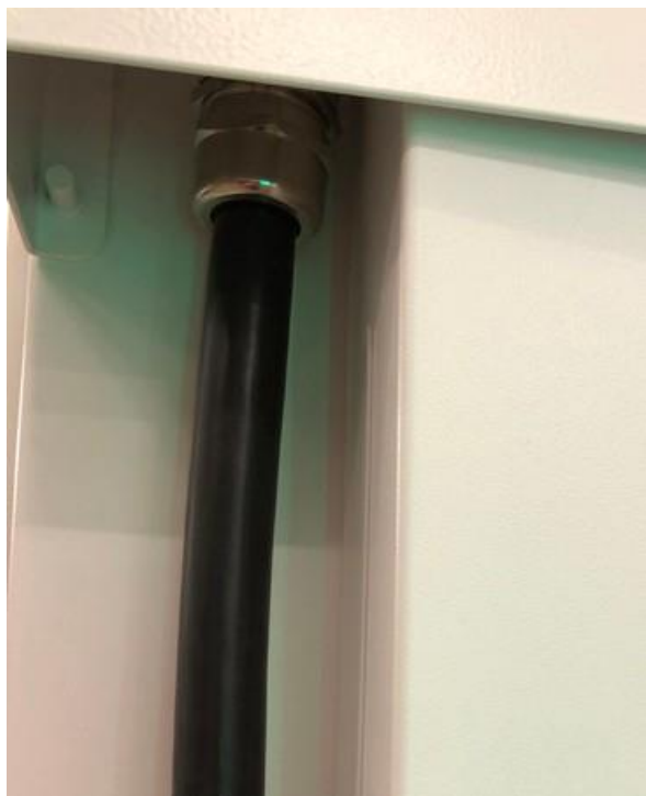
Kabelaustritt links (CCS)
